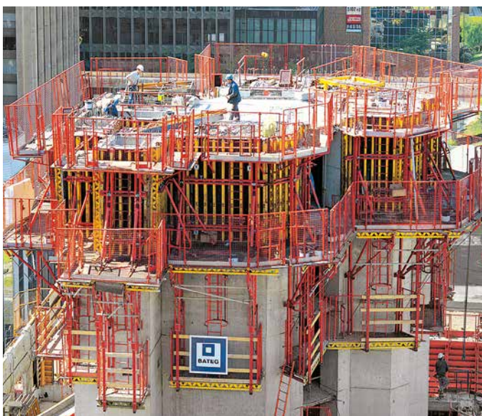
Multi-storey building in Paris with VARIO GT 24 and CB 240 climbing formwork systems.
