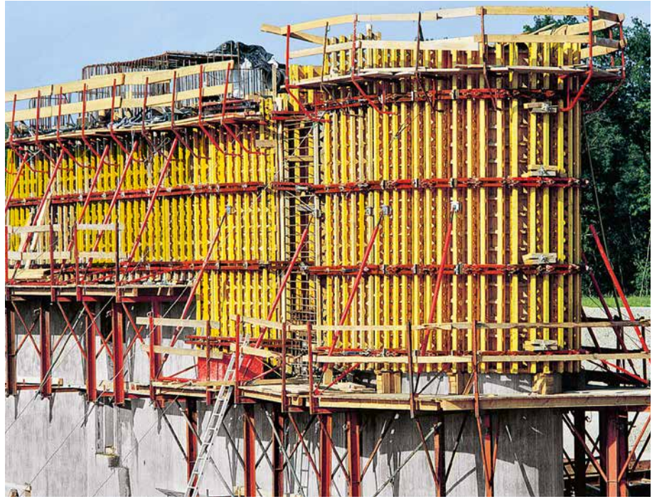
Front of the weir pier. VARIO in combination with GRV circular formwork system on KGF 240 climbing scaffold.
