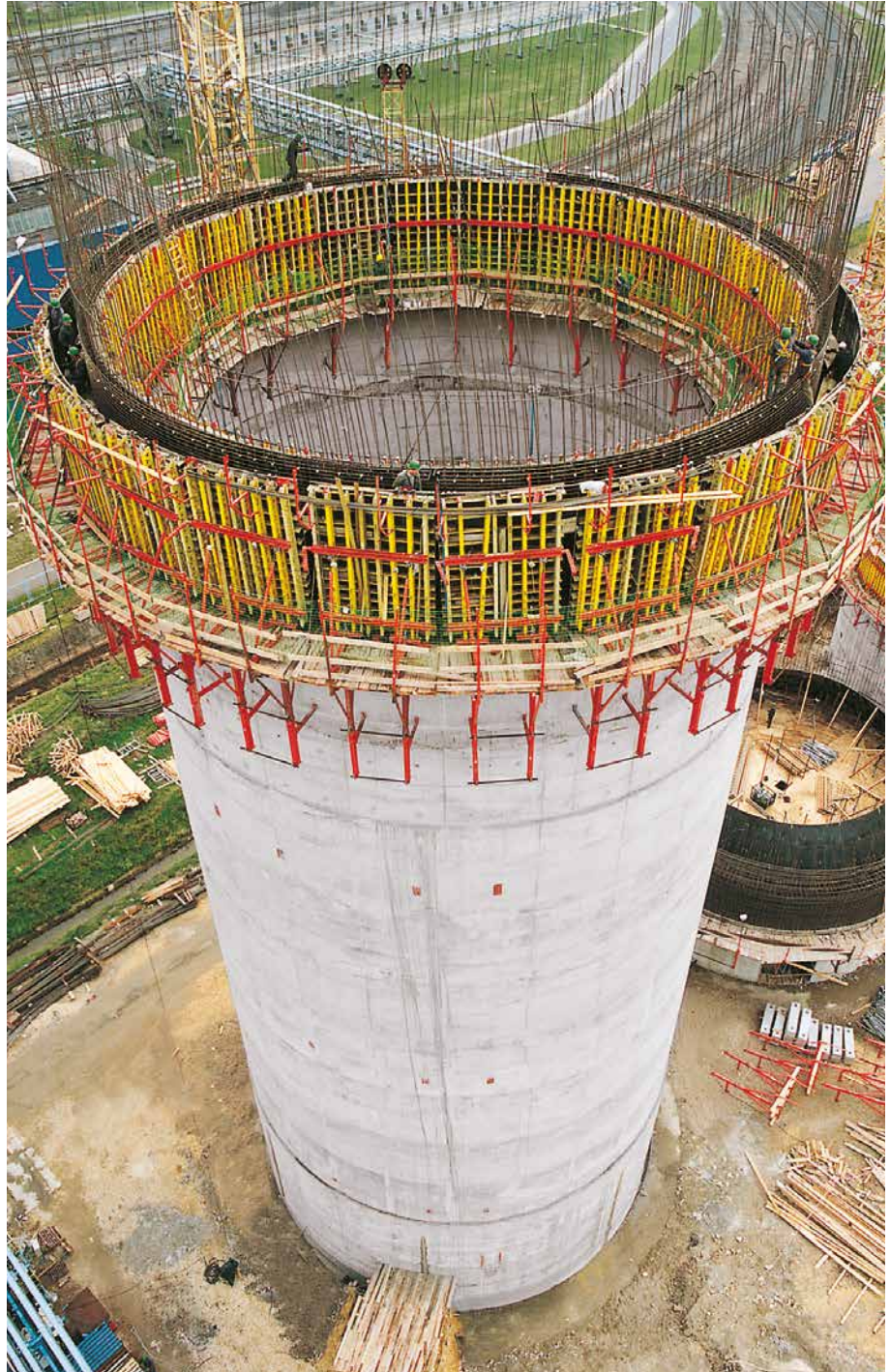
Silo, h = 72 m, Ø = 20 m for power station in Oppeln, Poland. Shuttered with circular VARIO girder formwork on KGF climbing scaffold.
